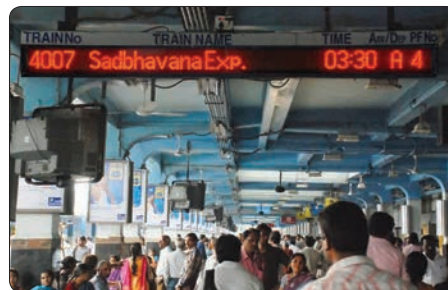
Single Line Display Installed at Secunderabad Railway Station
