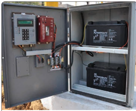
Wireless Master Control Unit
