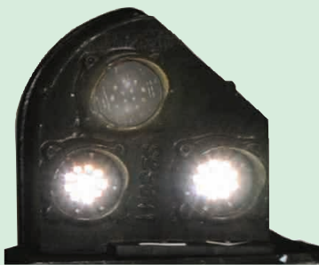
Position type Shunt Signal
